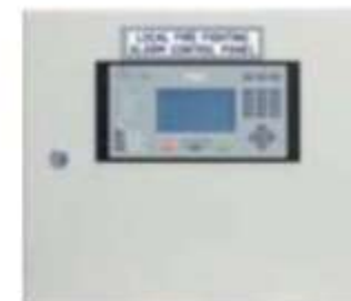
Alarm Control Panel
