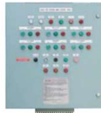
Main Control Panel
